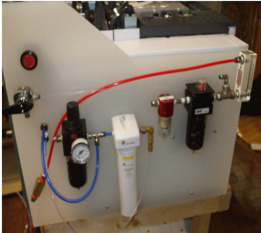
Figure 2: Custom sampling panel installed on mud logging G.C.
